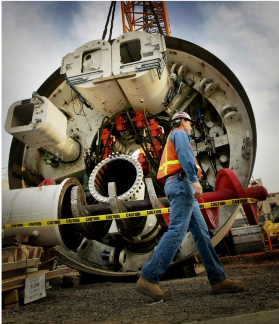
A construction worker walks past a massive tunnel boring machine at a Metro Rail construction site in Los Angeles in 2005.
